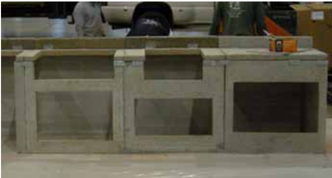
Step 7 - Mark and cut appliance openings to specifications of appliance manufacturer, using construction marker and standard masonry saw blades.
